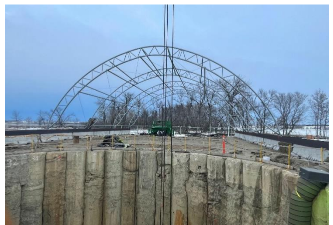
Winter Enclosure Structure
